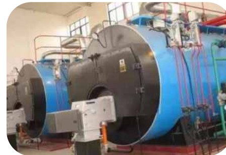
The boiler room
