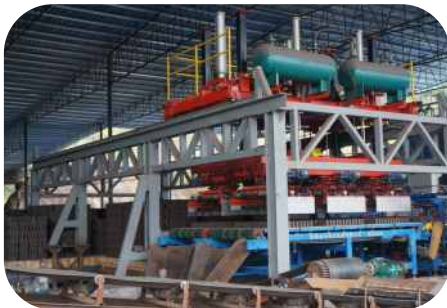
Bricks and tiles plant
